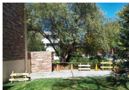
Cement was poured in mid-October to allow more bicycle racks to be added.
